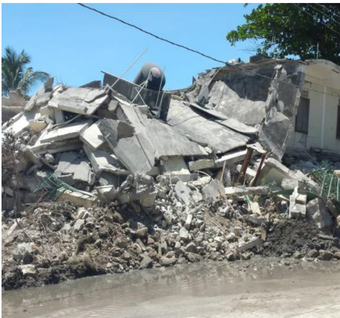
Collapsed house in Eveche du Sud © IOM 2021
